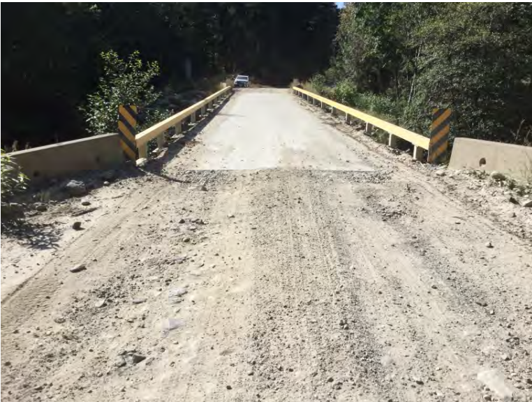
Potholes at approaches
