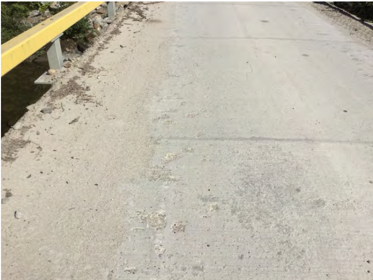
Track wear on wheel path
